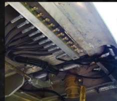
Central Grease Block and Floor Drain Valve
